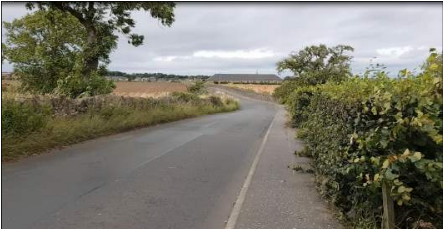
Photograph 3 - View along Dalmahoy Road towards culvert (at dip/bend in road) over unnamed watercourse under (flow from left to right)
